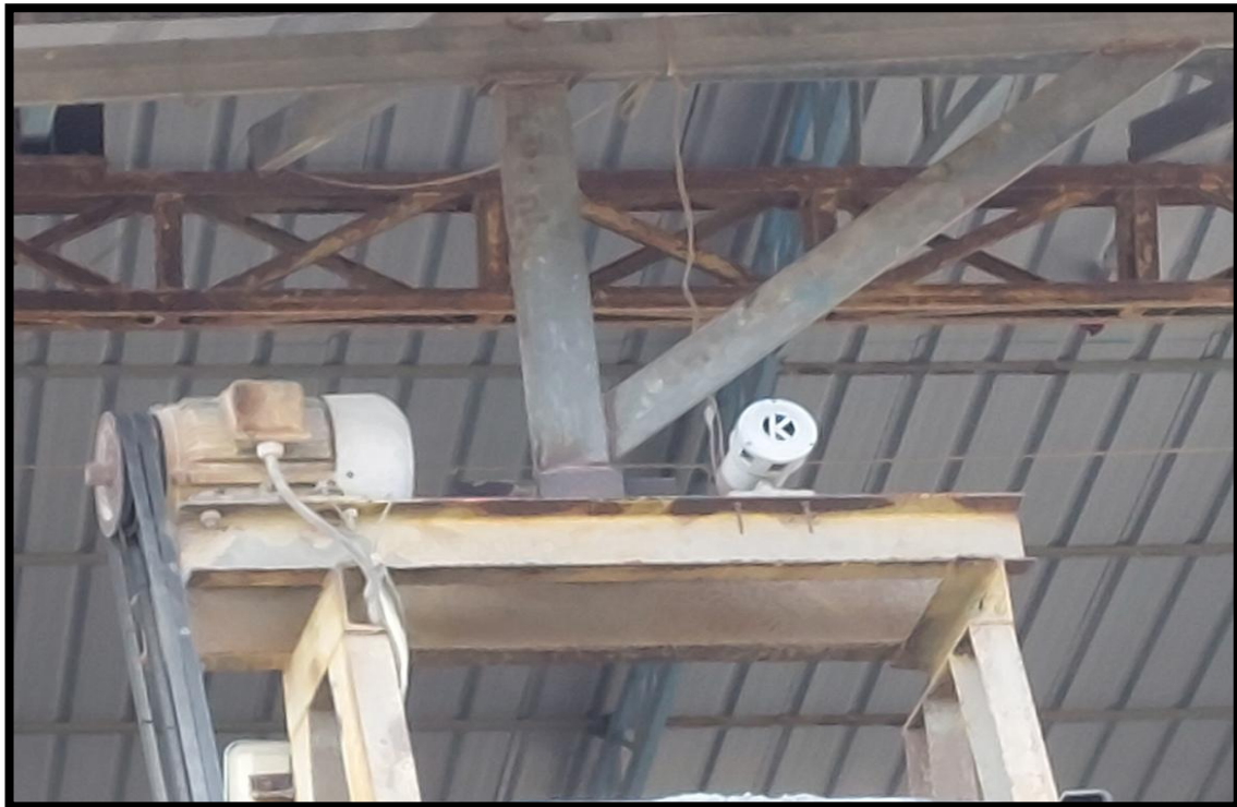
Warning alarm installed in the project site
